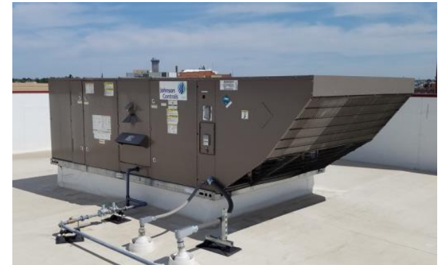
Roof Top Unit
